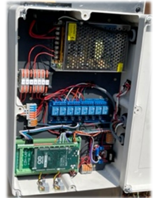
Shawnigan Waterworks filter cleaning machine (2022)
